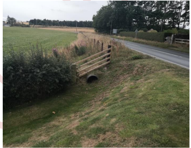
D4: - Existing culvert pipe for surface water run off from the field where the extended Car parking is planned
