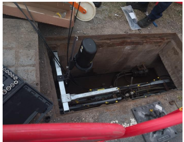
D6: - Telecoms trench on road outside of the Castle Lodge with water run-off at the bottom flowing North
