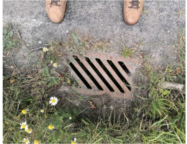
D2: - Typical surface water run-off drain on the road running down to the Castle Lodge & proposed visitor centre
