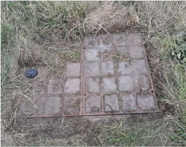
D3: - Typical sewer drain on the side of the road running down to the Castle Lodge & proposed visitor centre
